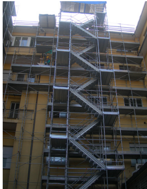
Temporary Multidirectional Staircase
