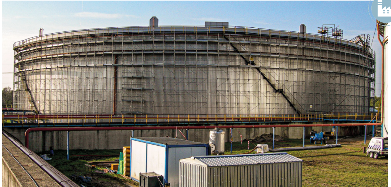
Edipower Power plant, Turbigo (MI)
